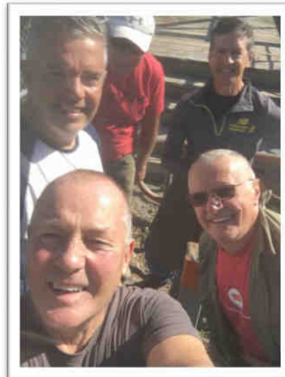
Alan Laver, Vince Zvonar, Jacques Boilard, Chuck Taylor, and Rick Waters during installation of posts to restrict motorized vehicles from going over the pedestrian bridge at the QEW. Four posts and 660 lbs of concrete mix and some heavy slogging.
